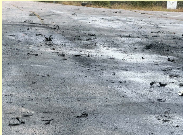
Photo of road damage due to stunt driving
